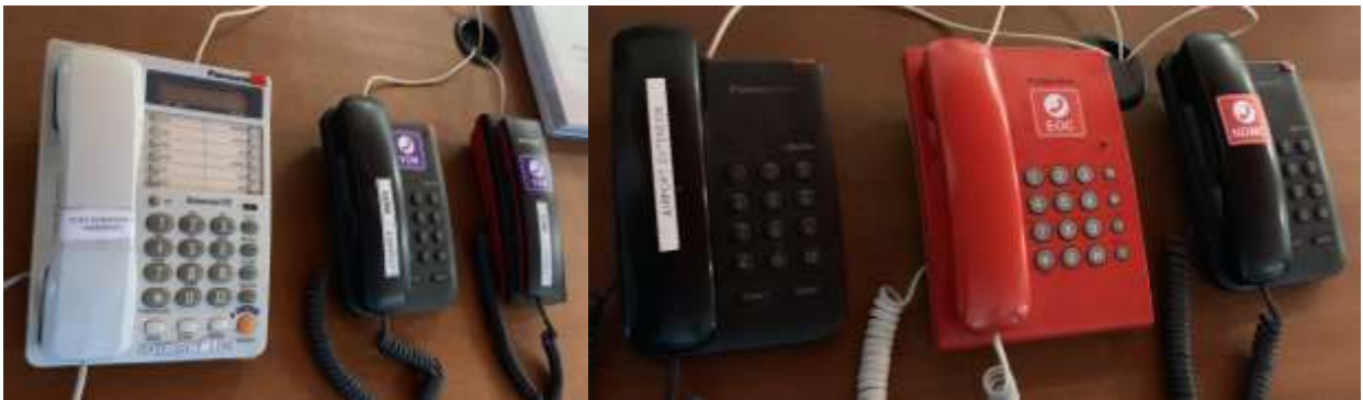
Figure 03: Dedicated Land Phone Communication system Maintained
